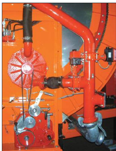
Electric valve motorisation
